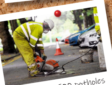
More than 5,500 potholes fixed and road improvements for every community in our £5m highways programme
